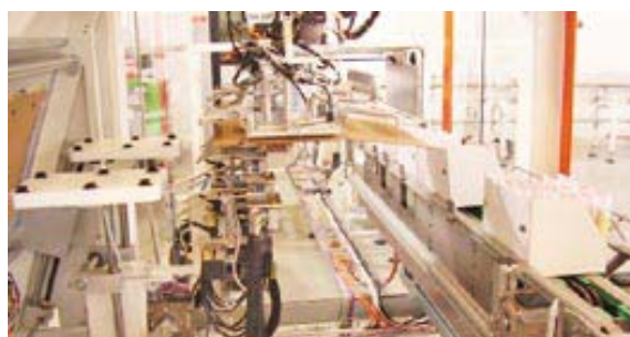
Station de couvrage
